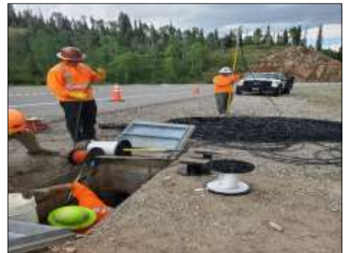
During the 2023 work season, an installation crew pulls fiber optic cable through recently buried conduit along US 160 Wolf Creek Pass east of Pagosa Springs. Courtesy photo.
