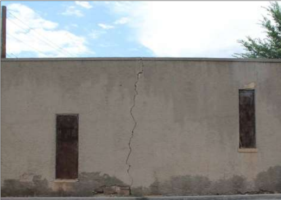
The west wall of the Montrose County Jail built in 1885, and still standing, shows the steel mesh screens that were used in place of windows and bars. The jail was known for years as "The Tin Can Jail." Photo by Bob Cox
