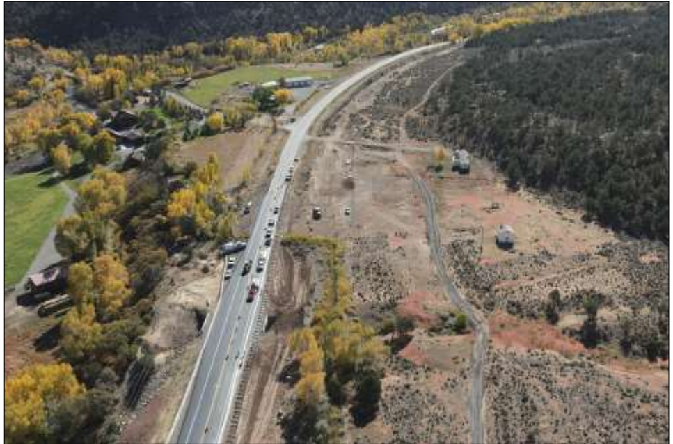
Crews made wildlife and mobility safety improvements to an eight-mile section of US 550 bordering Ridgway State Park from Mile Point 109 to 117. CDOT courtesy photo.
